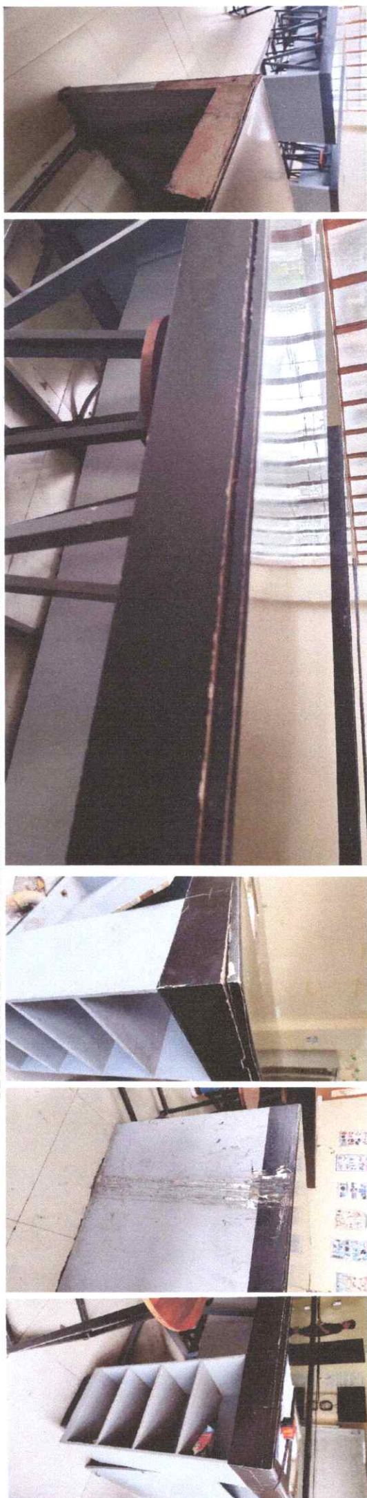
TAINED PAINTS, CRACKS AND DAMAGED CABINET ON LABORATORY TABLES NOTE: FOR REPAINTING AND REPAIR OF TABLES
